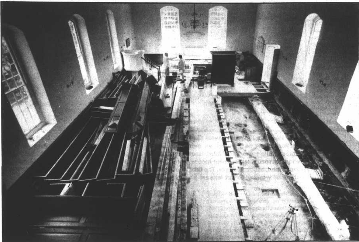
Workers stacked pews on either side of the church to get to the floorboards to remove then and replace damaged joists and boards. (Stephen M. Katz photo)
